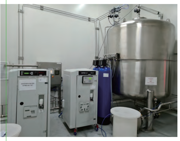
Lipa — Water filtration system.
